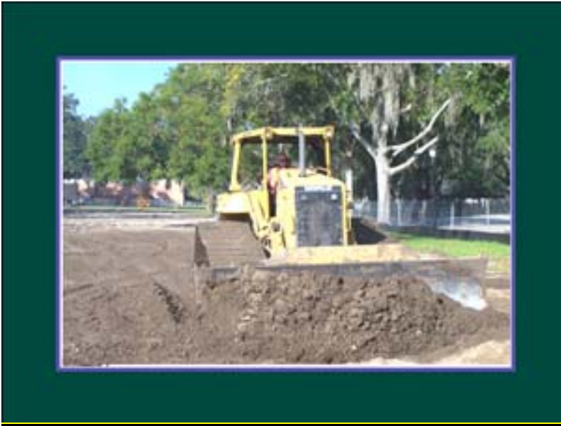
In October 2008 the first bulldozers and backhoes arrived on campus for site work.
